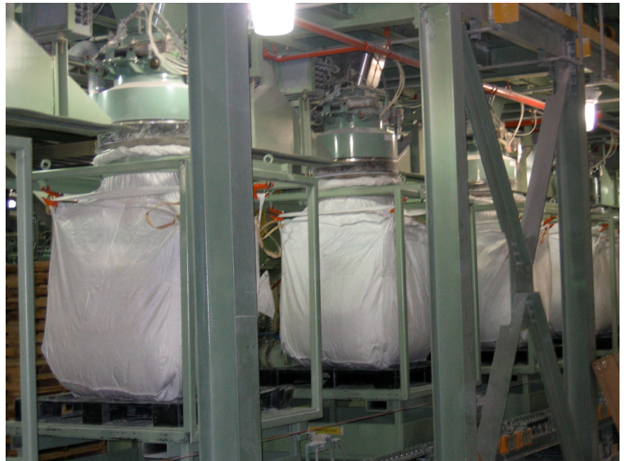
Minerals processing facility—bulk bagging system
