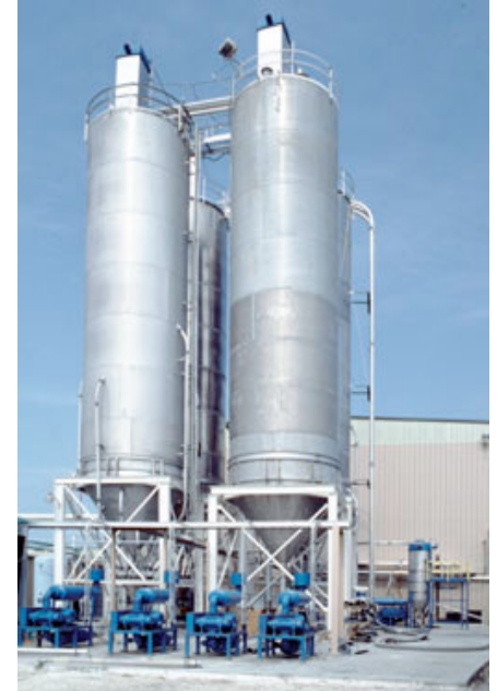
Plastic manufacturing facility -- silos with pneumatic conveying
