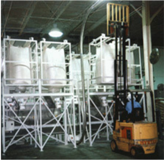
Chemicals facility—discharging and metering bulk raw materials into process
